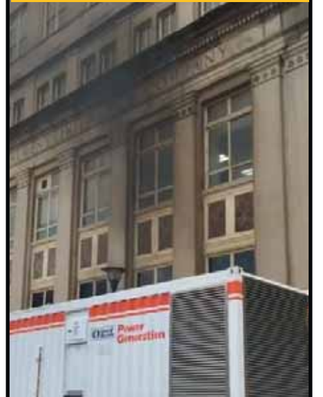
A generator fire was just one of the issues plaguing the former Division of Welfare headquarters in Newark. Photo via Facebook
